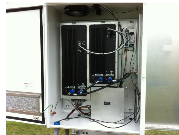
7. Inside Control Enclosure
